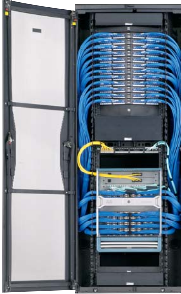
(Nexus 7009 "Heavy Copper" Pre-Configured Physical Infrastructure shown)
