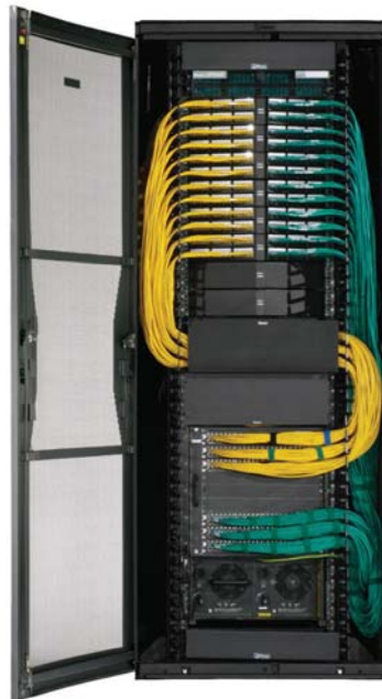
(Catalyst 6509 "Heavy Copper" Pre-Configured Physical Infrastructure shown)
